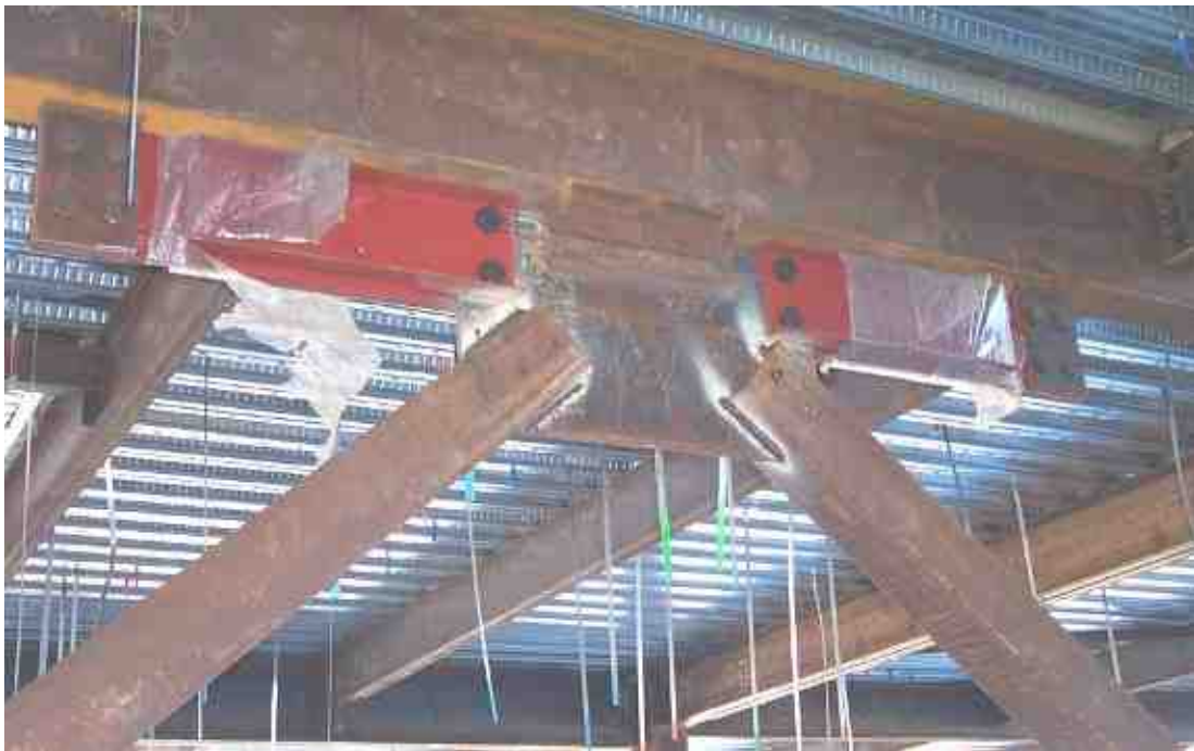
Figure 5. Typical Chevron brace with two friction dampers at the apex (during construction)
